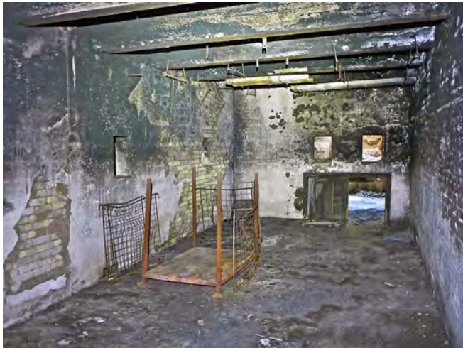
Fire-damaged West Battery Magazine, Windmill Hill
